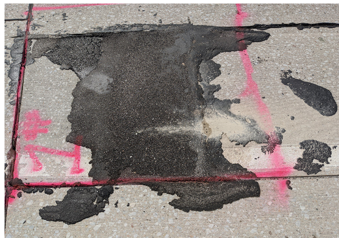
Pavement Design observed 4'x4' patches failing prematurely.
