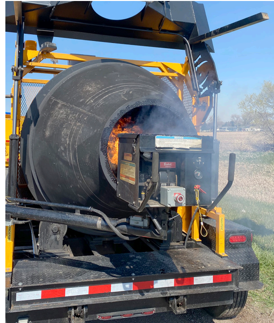
Flexible Pavement Section uses a portable asphalt recycling machine to patch asphalt pavements during cold weather.
