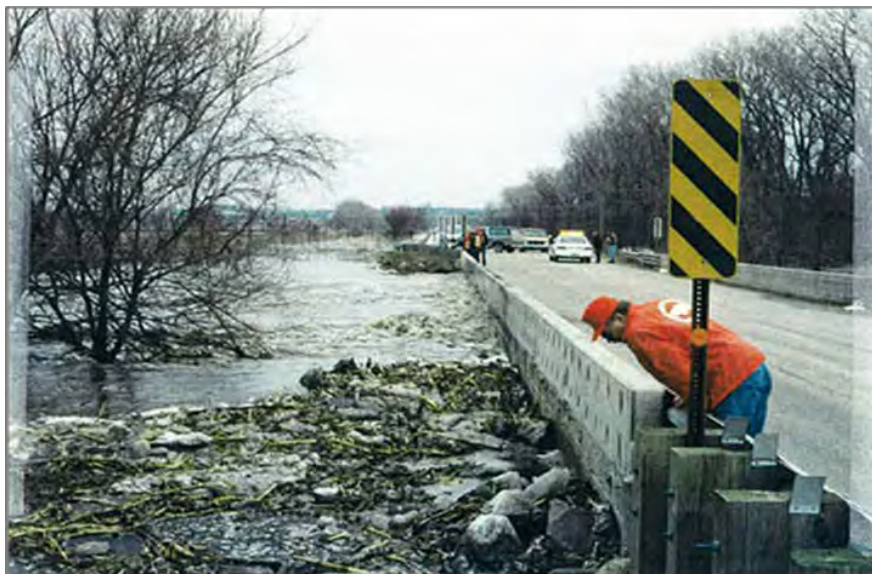
Overflow bridge flowing full due to ice condition
