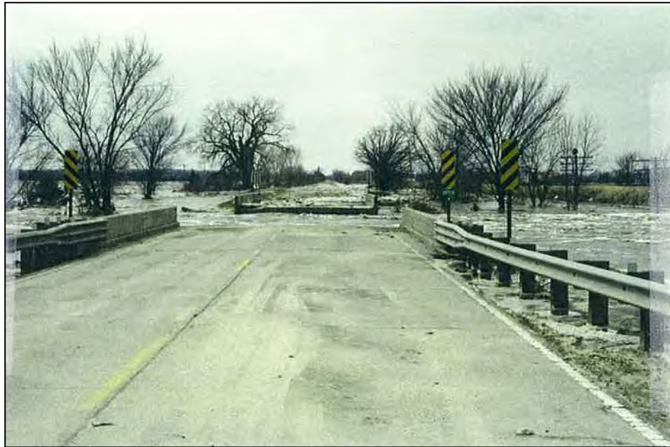
Overflow bridge failure due to high flows under bridge shown above
