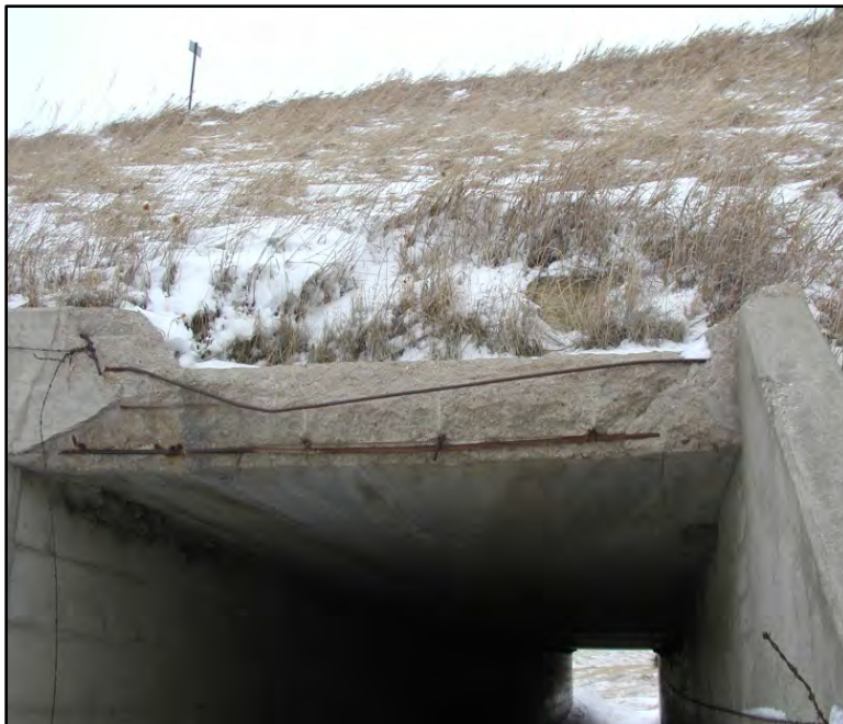
Item 324 Code: 4 POOR CONDITION Description: Large spall, Exposed Rebar
