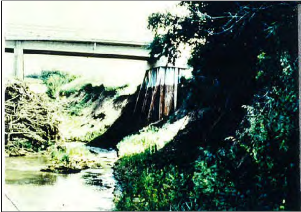
Debris trapped at pier
