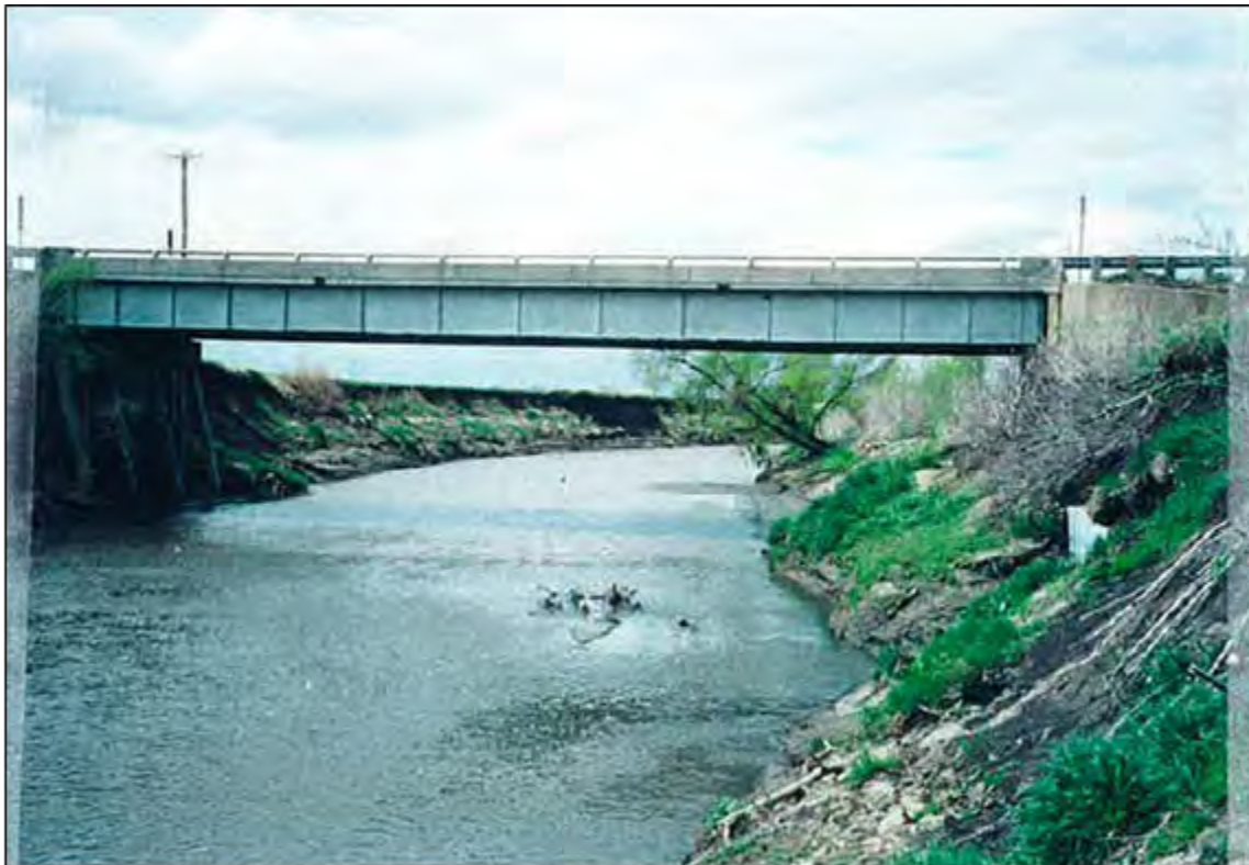
Bridge with inadequate length
