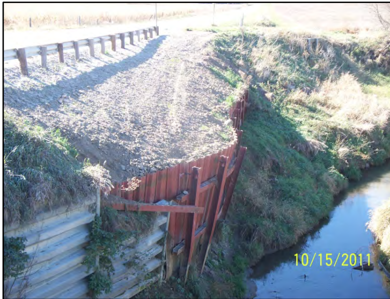
Item 326 Code: 6 SATISFACTORY CONDITION Description: Embankment is beginning to slump, protection is strained
