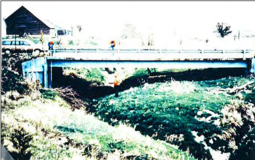
Bridge opening partially silted shut from aggradation
