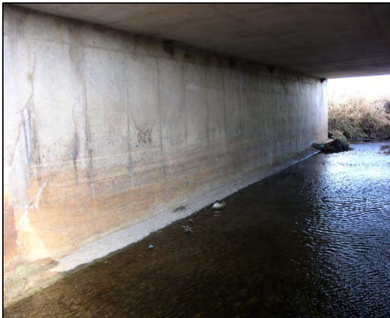
Item 323 Code: 7 GOOD CONDITION Description: Minor cracking, Light Scaling
