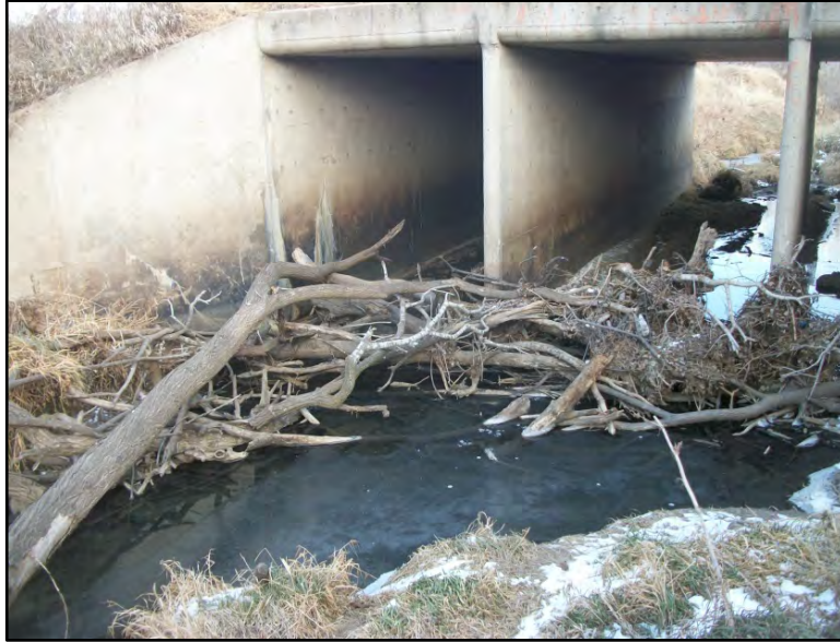
Item 325 Code: 5 FAIR CONDITION Description: Trees and brush restrict the channel
