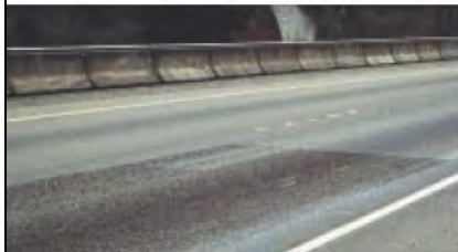
Chip Seal Repair Low
