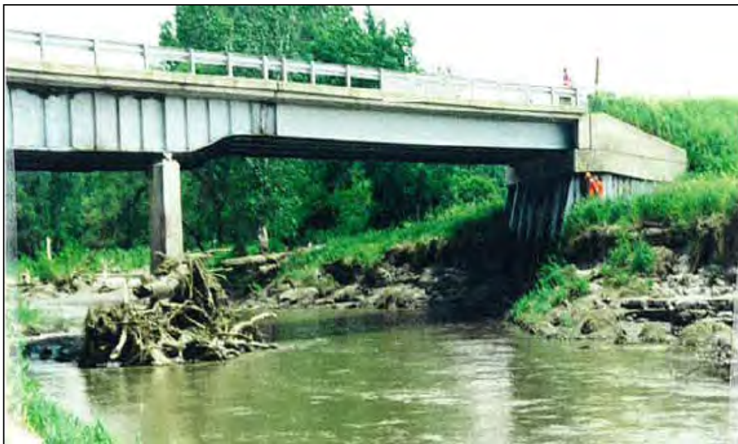
Stream meander attacking abutment
