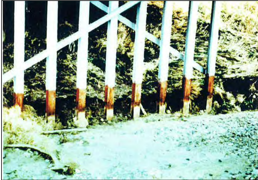
Portion of a bridge bent exposed due to degradation
