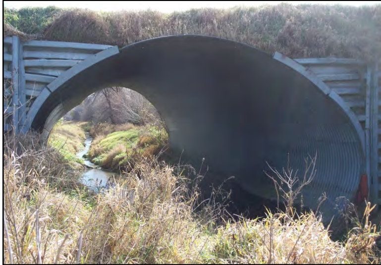
Item 323 Code: 5 FAIR CONDITION Description: Distortion in the far upper left end section of culvert
