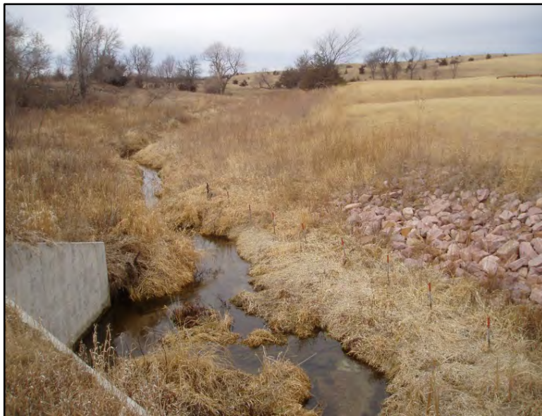
Item 327 Code: 3 SERIOUS CONDITION Description: Poor alignment even with skewed barrels
