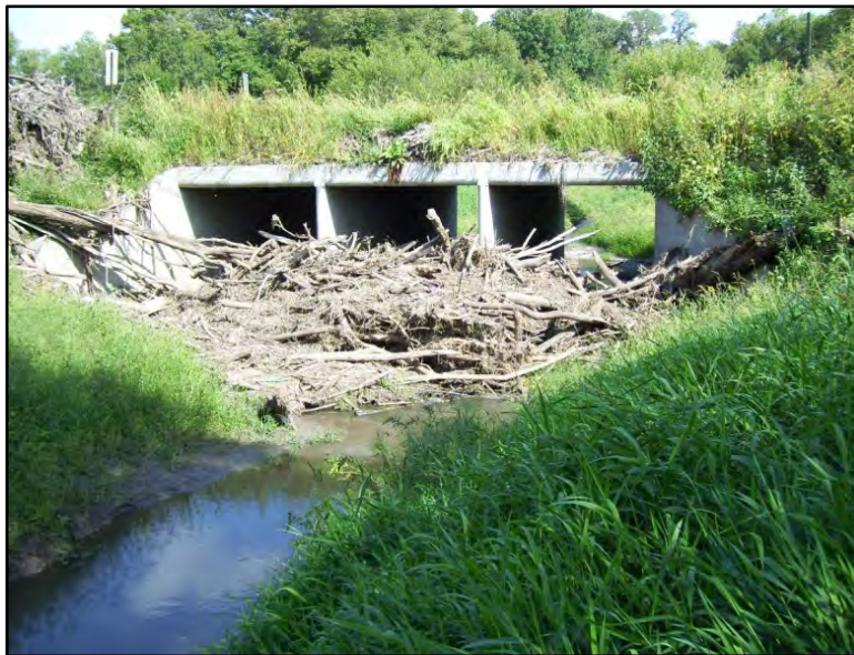
Item 325 Code: 4 POOR CONDITION Description: Large deposits of debris in the waterway blocking inlet
