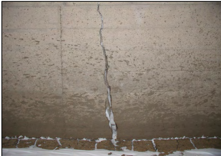
Item 323 Code: 4 POOR CONDITION Description: Wide Crack
