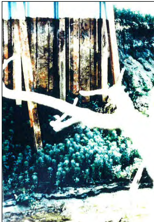
Undermining at a bridge abutment
