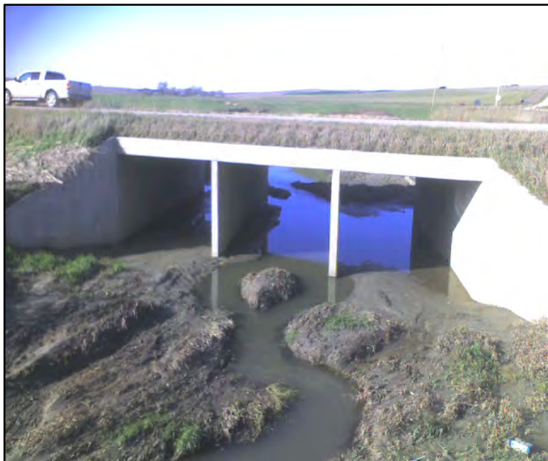
Item 329 Code: 0 Description: Smooth transition out of culvert, No drop at outlet
