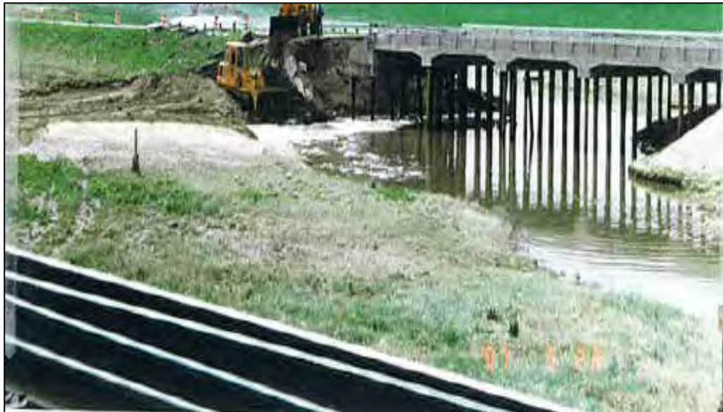
Abutment failure due to improper skew
