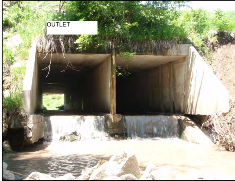
Item 324 Code: 3 SERIOUS CONDITION Description: Settlement of wing footing and undermining
