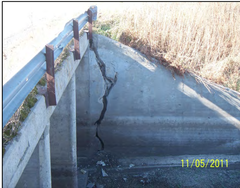
Item 324 Code: 3 SERIOUS CONDITION Description: Wingwall nearly severed
