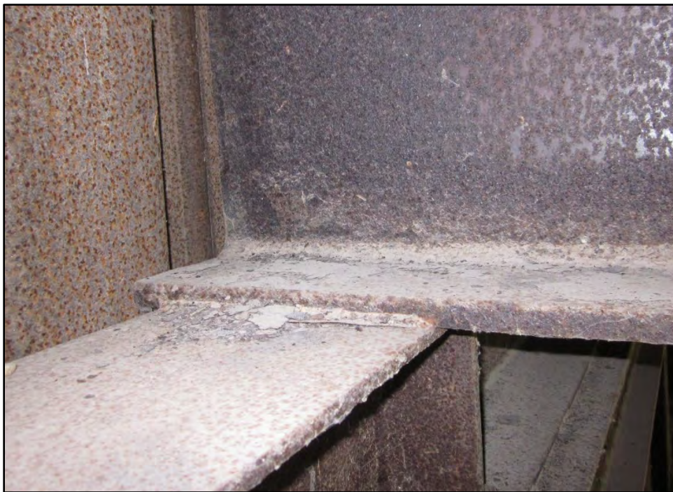
Item 311 Code: N not applicable Description: Stringer is welded to cap. There is no bearing device
