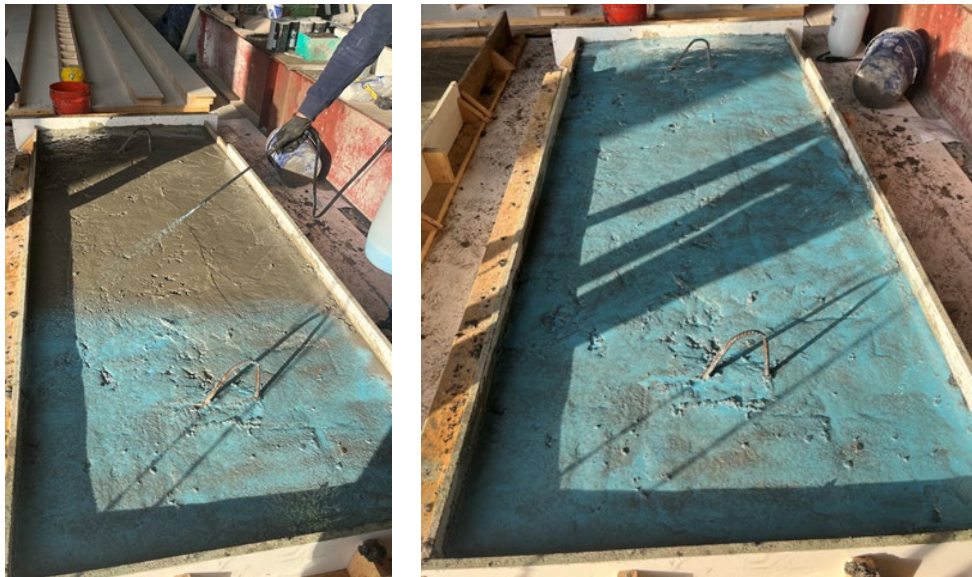
Figure 6.3 Application of Top-Cast surface retarder (Blue) from Dayton Superior on fresh concrete.
