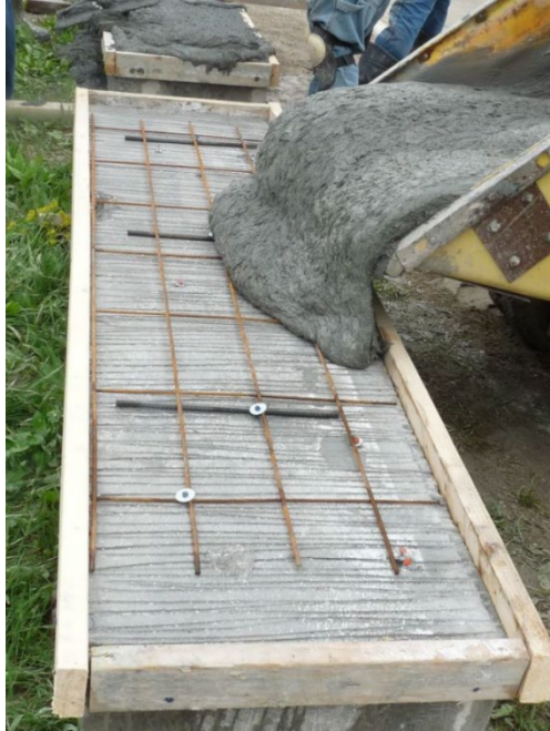
Figure 2.18 Surface preparation on concrete deck used for slab specimens (Wibowo et al., 2018).
