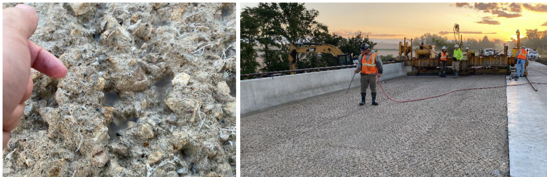
Figure C.2 From left to right: wet surface; removing excess water by air-blowing before the UHPC placement (SSD condition).
