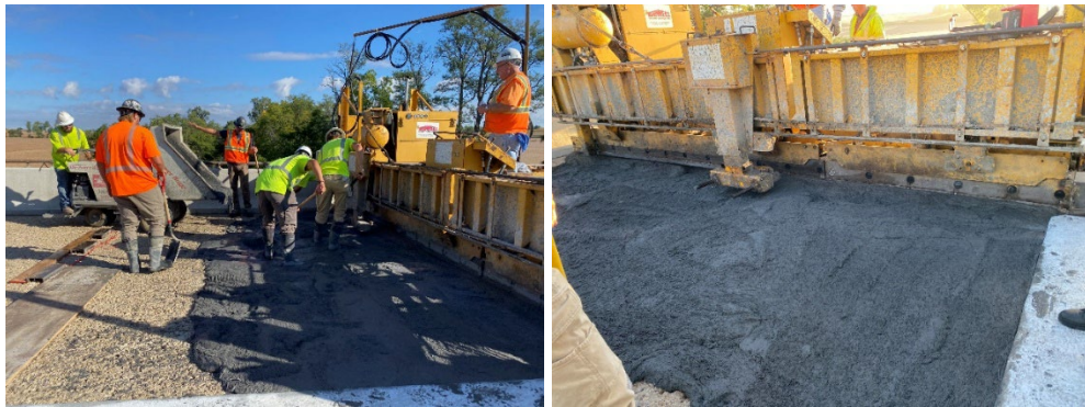
Figure C.7 From left to right: UHPC overlay installation and consolidation with a paver; Spread of material before consolidation.
