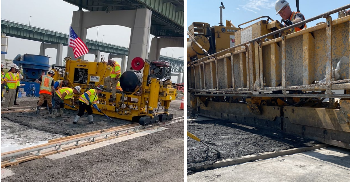
Figure 7.2 Examples of UHPC Overlay Mockups (Left: from 2023 UHPC Symposium; Right: from 2024 IADOT Cass County Bridge Overlay Project)
