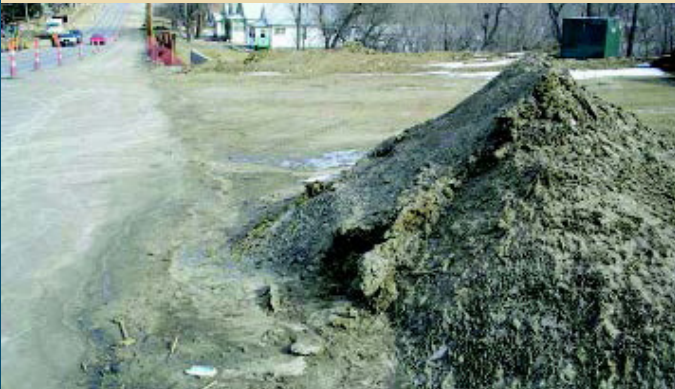
Pictured: Poor example of stockpile management. Protect stockpiles with silt fence or other BMPs and seed if left undisturbed for more than 14 days.
