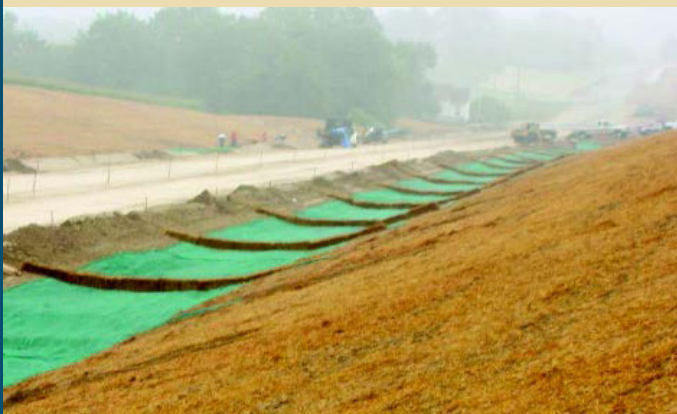
Pictured: Good example of TRM installation in a channel with mulch on the backslope.
