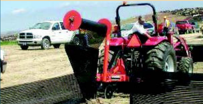
Pictured: Good example of silt fence installation using a silt fence plow on a tractor.
