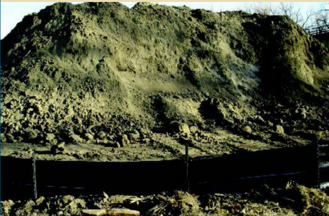
Pictured: Good installation of silt fence around stockpile. The fence is placed at least 6 feet from the toe of the slope to provide a catchment area and easy clean out. Stockpiles must be stabilized if left undisturbed for more than 14 days.
