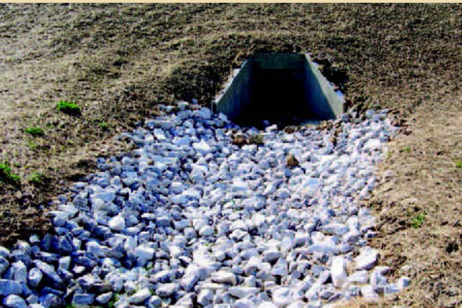
Pictured: Outlet is protected with riprap and adjacent areas are mulched and seeded to prevent erosion. Additional barriers around outlet could prevent sediment from getting into the channel until final stabilization is established.
