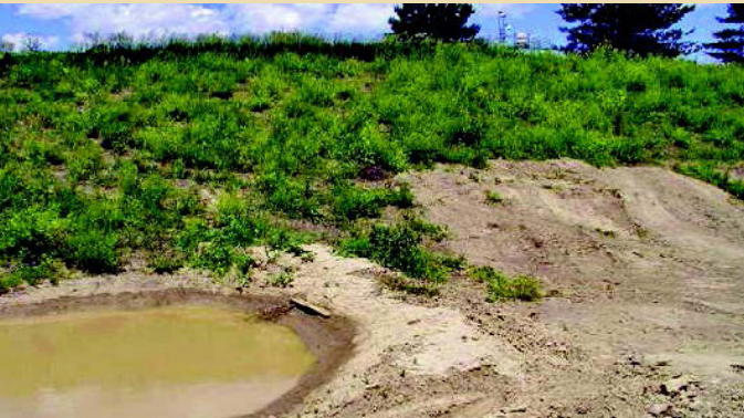
Pictured: Good example of an earth check that can be cleaned out easily.
