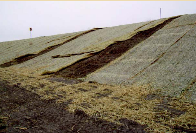
Pictured: Poor Erosion Control Blanket installation. Blankets were not anchored properly and need to be repaired.
